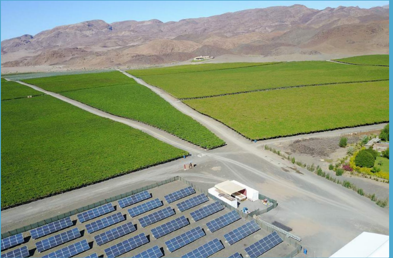
Silverlands Vineyards makes the most of the desert sun in southern Namibia with a 210 kW solar power unit. This reduces dependence on fossil fuel generated electricity, and de-risks the farm in the event of power cuts on the main grid.
