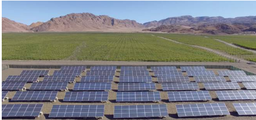
The 210 kW solar power unit at Silverlands Vineyards in Namibia.
